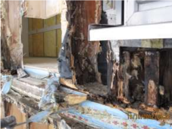
Fig. 1 Moisture caused damage at exterior wall resulting from leaky sill connection.
