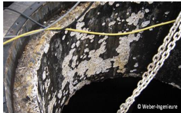
Figure 1. Concrete corrosion within a digester.
