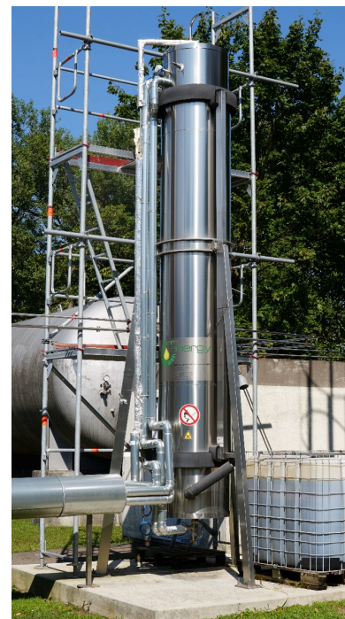
Figure 16: Pilot-scale reactor at the wastewater treatment plant Garching.
