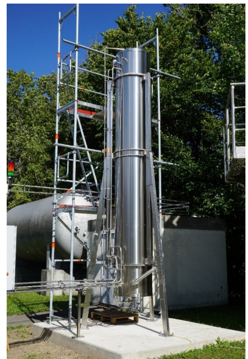
Figure 12: Pilot-scale reactor at the Garching wastewater treatment plant.
