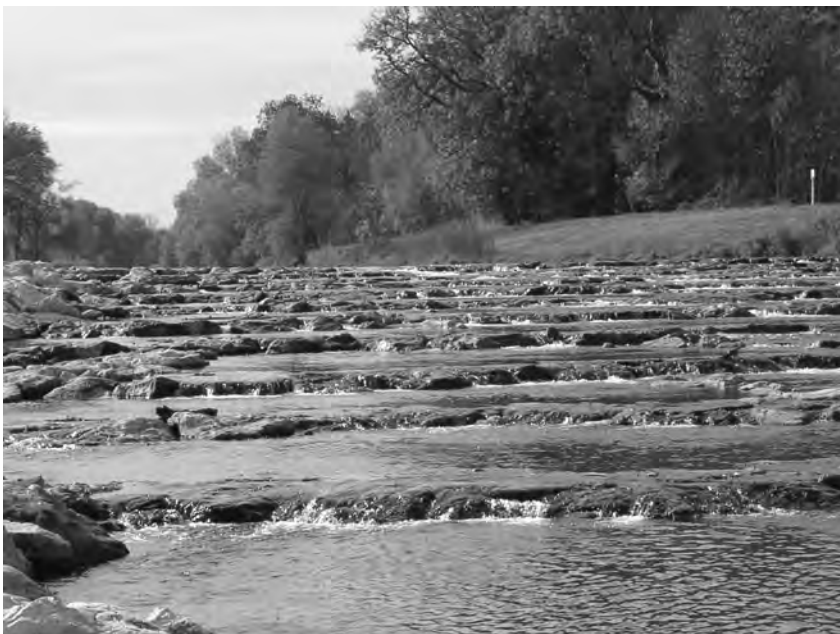
Fig. 4.4.6: Bottom ramp Kolbermoor in the river Mangfall, photo made on Oct.25.2006, Q = 4.84 \text{ m}^3/\text{s} ( Q_{30} )
