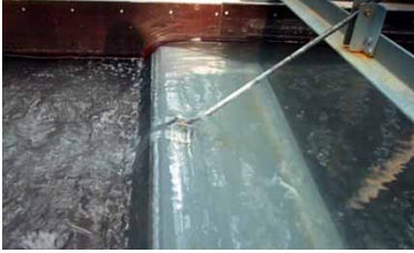
(a) BP 1 : Gate 5 cm overflowed
