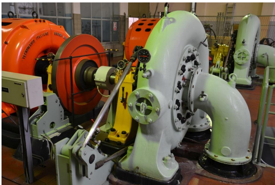
Fig. 1 Small HPP Hubelj machine room. Measurements were performed on the smaller turbine in the back of the machine room (P = 900 kW).
